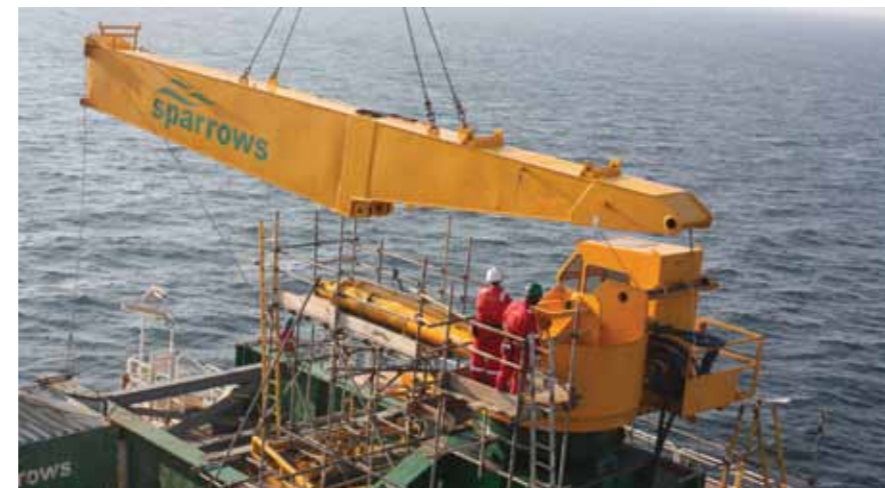
The DOL-1 platform and the modular crane
