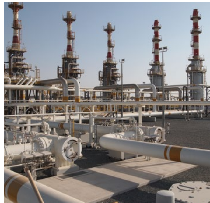
The five heaters that were inspected
