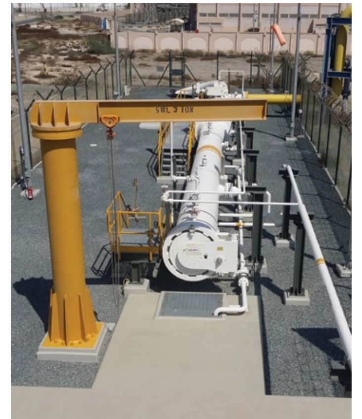
The new pigging facility will ensure uninterrupted gas supply to our customers
