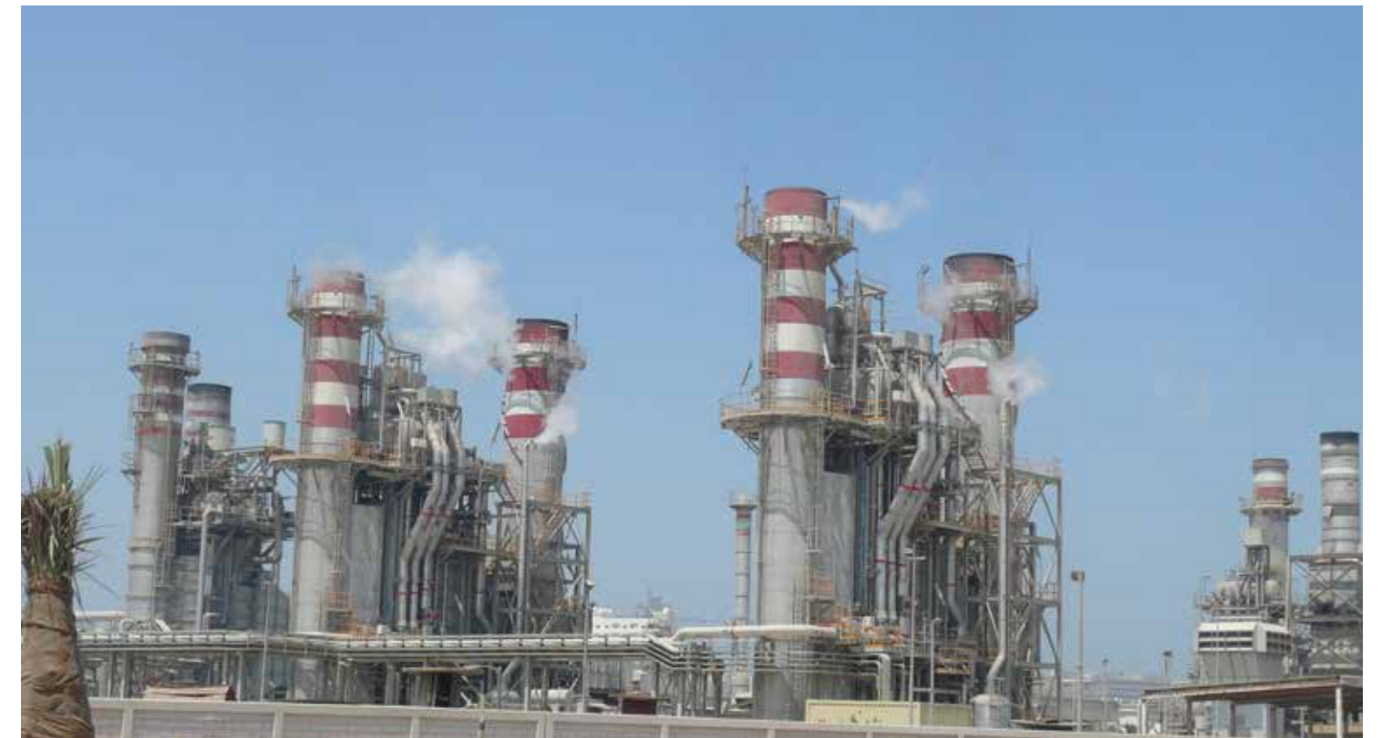
Turbine & Desalination Plant, Nakheel- Ras Al Khaima
