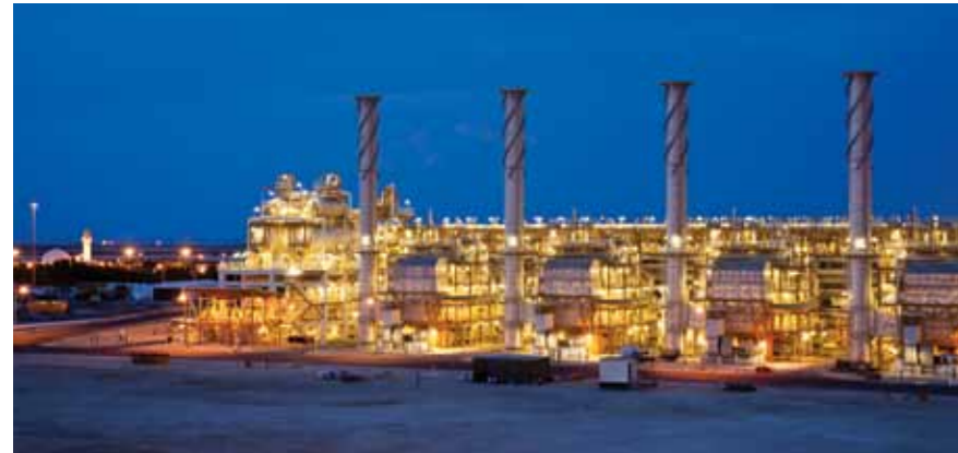
Dolphin Energy's gas processing plant at Ras Laffan, Qatar
