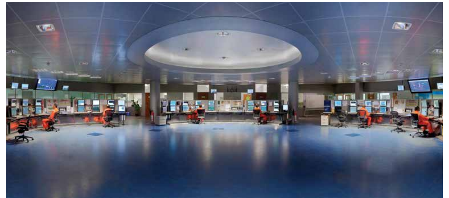
Our control room in Ras Laffan helps to power the performance of the company
