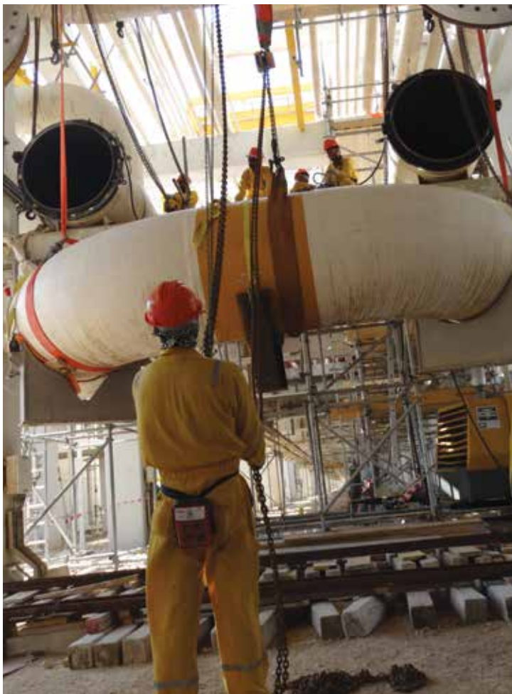
Removal of the 48" spool from the compressor suction header, prior to replacement with the new spool
